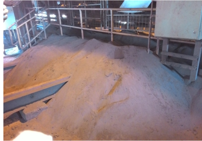
Spillage from conveyor DPC3 skirt area
