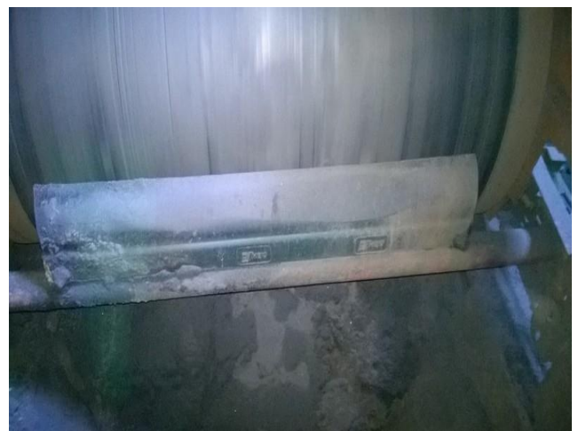
Condor HR Cleaner installed on the belt
