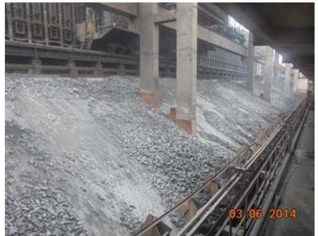
Belt carrying hot coke. Notice blisters on the belt surface
