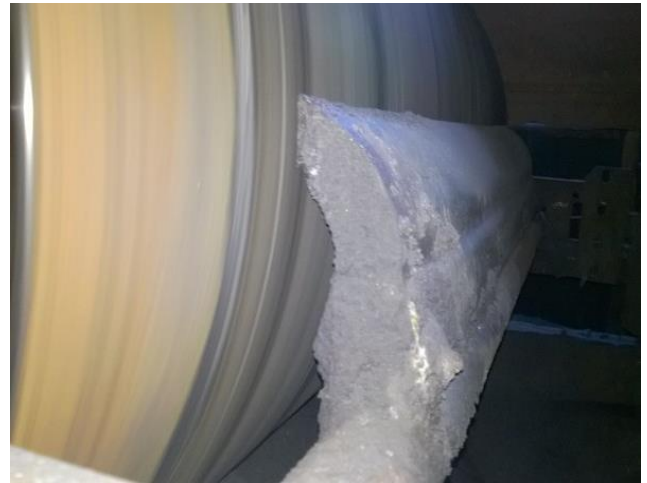
Condor HR cleaner installed on the belt- view from side
