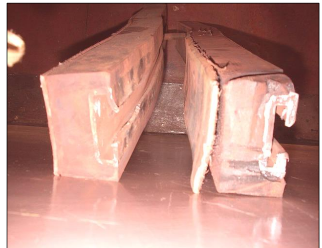
Damaged Impact Bars
