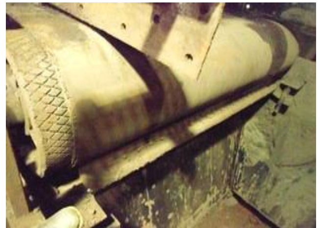
Cleaner used previously. Note material build-up on the frame due to the faulty design
